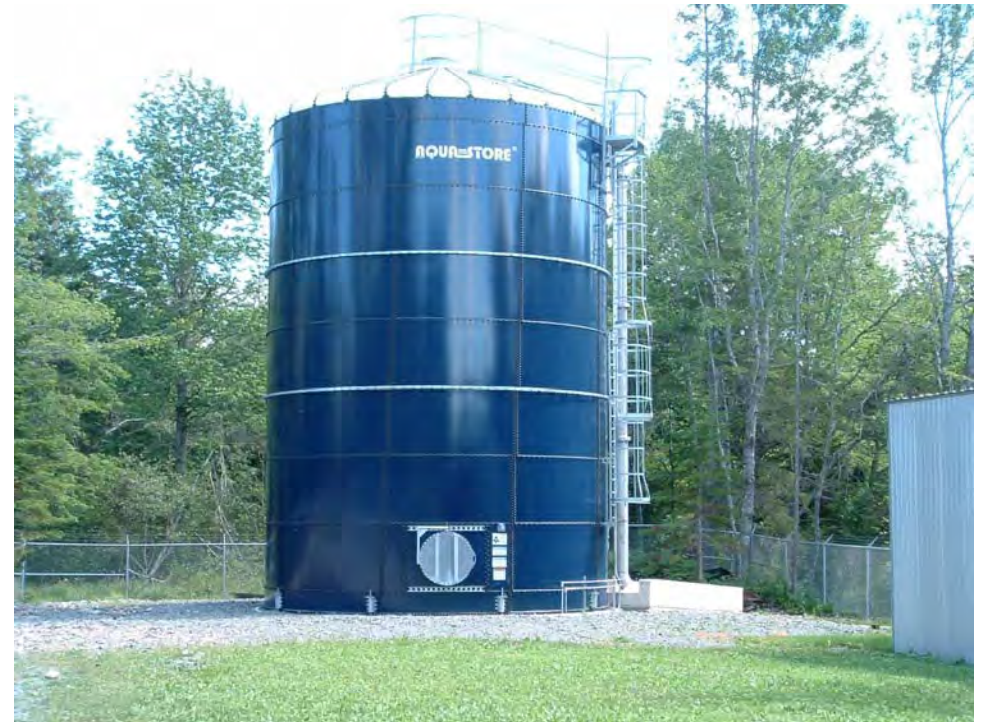
Above Grade Bolted Steel Tank
